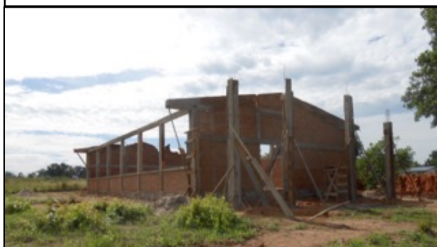
IMCK’s college, called ISTM, has this new building under construction. This is a large classroom that will also serve as an auditorium.
