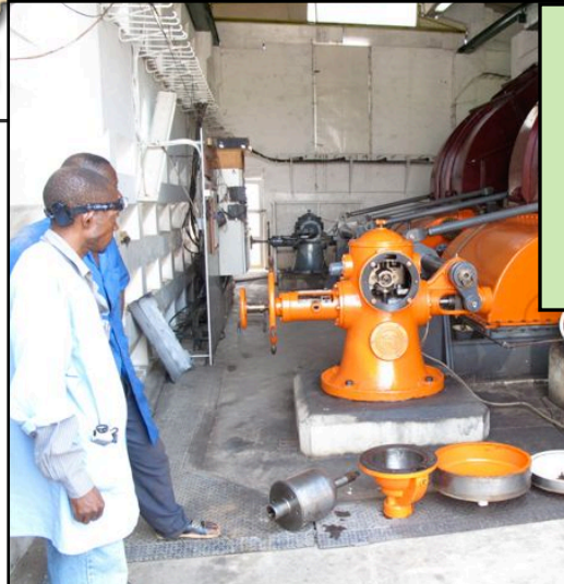
Nkashama Muyembi (Electrician) and Ntefu Kabemba (Chief of Hydro) regard the G2 governor, where the problem exists.
